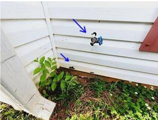
Photo 4-2 Minor damages noted in some areas The hose bibb inoperable and should be secured to the home
