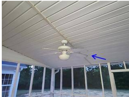
Photo 24-2 Screened in porch ceiling fan appears inoperable
