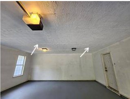
Photo 6-2 Repairs noted in some areas of the garage ceiling. The area was dry at the time of the inspection. Recommend monitoring
