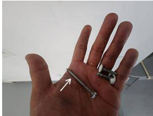
Photo 9-2 Some panel screws are missing - One incorrect (pointed) screw used recommend replacing as needed
