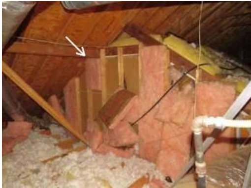
Photo 26-3 Insulation fallen in some areas above the living room. Also noted with the thermal camera
