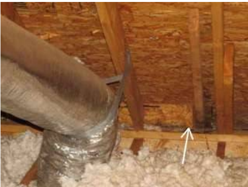
Photo 26-10 Dry stains chimney area
