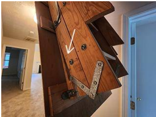
Photo 26-1 Attic stairs damaged
