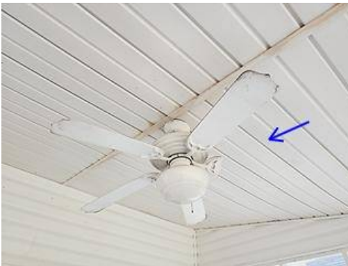
Photo 4-10 Ceiling fan damaged
