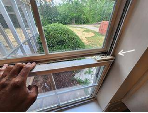
Photo 7-1 Kitchen sink window loose on the right-side
