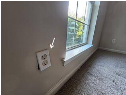
Photo 24-3 Some outlet covers are loose, recommend securing as needed - Front bedroom
