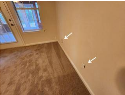
Photo 24-4 Outlet covers loose, master bedroom
