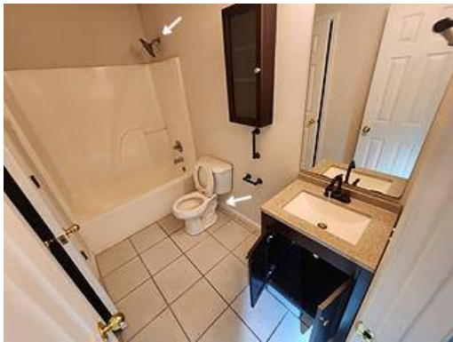
Photo 23-1 Hall bathroom toilet and showerhead are loose
