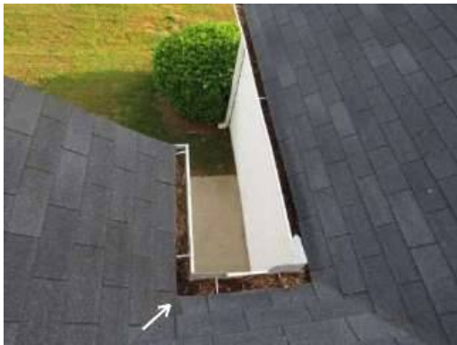
Photo 5-1 Some gutters are full, recommend clearing as needed
