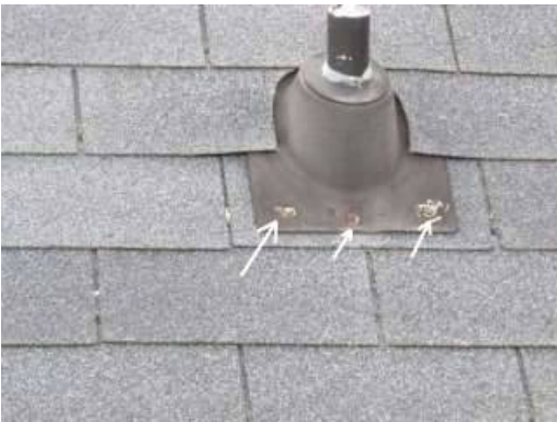
Photo 5-2 Nail heads exposed at some areas, recommend applying sealant as needed
