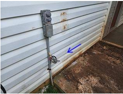
Photo 4-7 Wire splices exposed at exterior
