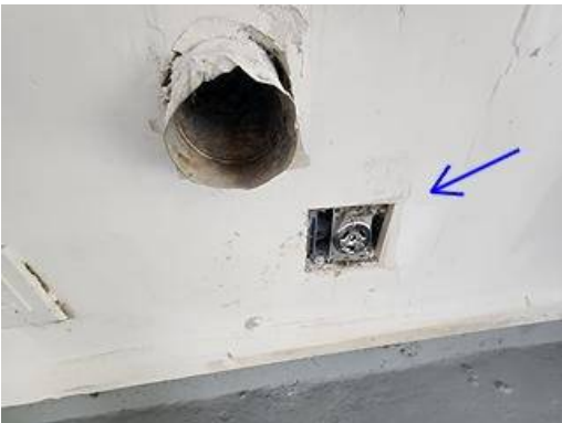
Photo 23-6 Dryer 3-prong, most new outlets are 4 prong. Dryer outlet cover missing
