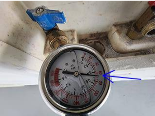
Photo 27-4 Water pressure @ 70psi
