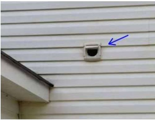
Photo 4-8 Exhaust cap damaged/missing
