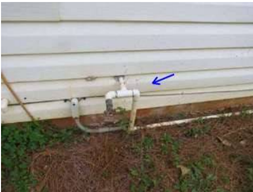
Photo 4-9 Hose bibb loose and should be secured, severe movement can cause leaks
