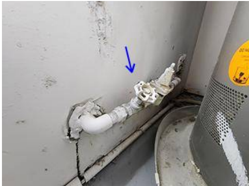
Photo 27-3 Garage shut off location
