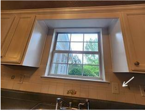
Photo 7-2 Right side sink switch did not operated anything, recommend evaluation
