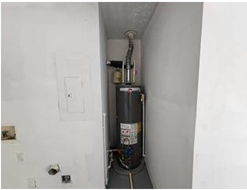
Photo 14-1 Rheem gas water heater Garage location
