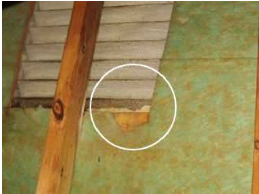
Photo 26-5 Gable screen damaged
