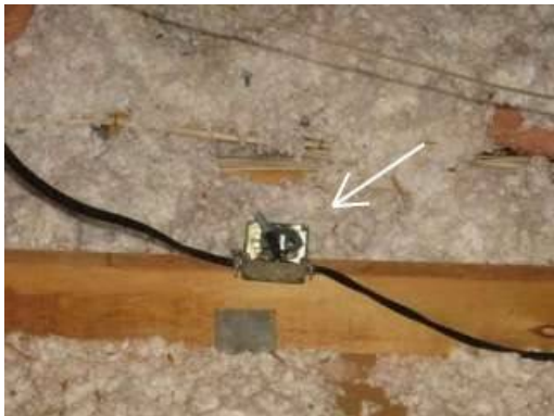
Photo 26-9 Exposed splices noted in some areas
