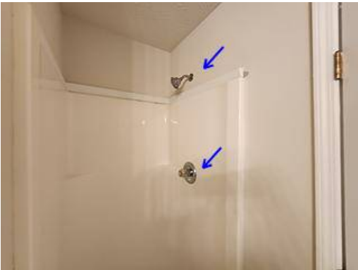
Photo 23-4 Shower head and handle loose in master bathroom
