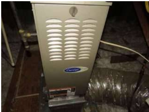
Photo 18-3 Carrier air handler unit Attic location
