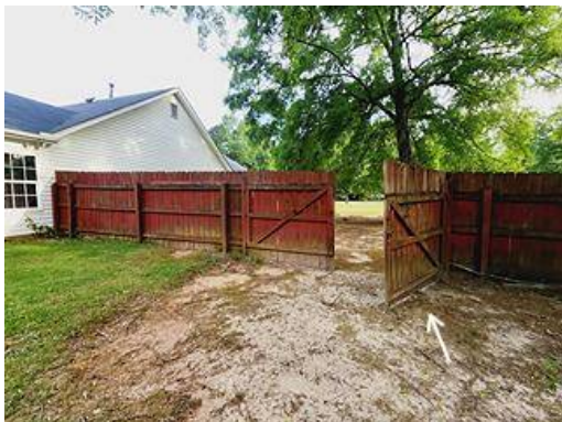
Photo 4-3 Both left and right gates are deteriorated and difficult to close
