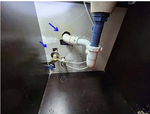
Photo 23-2 Recommend sealing all openings below hall sink
