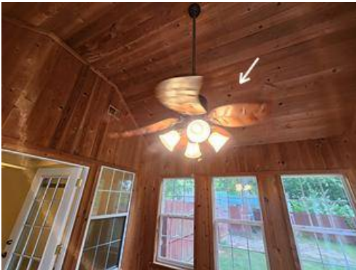
Photo 24-1 Sunroom ceiling fan wobbly
