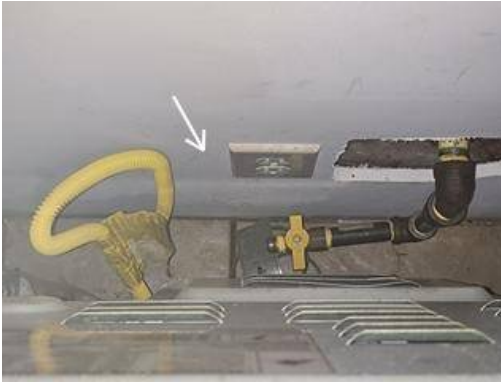
Photo 7-4 Unplugged, gas disconnected, exposed gas valve should be capped
