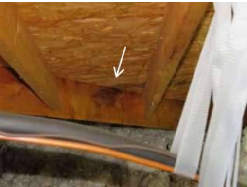
Photo 26-2 Dry stains noted in some attic areas. These areas were dry at the time of the inspection. Recommend monitoring in the future and if necessary have a qualified contractor evaluate and make any needed repairs
