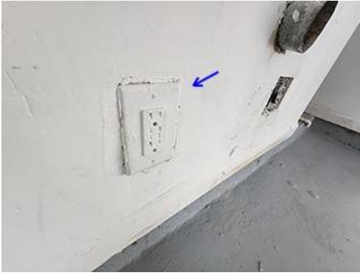
Photo 23-7 Laundry GFCI outlet loose
