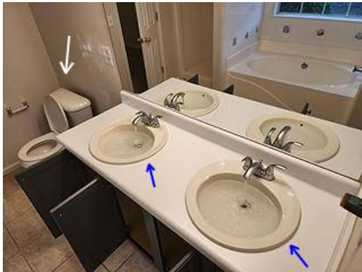
Photo 23-3 Master bathroom toilet loose The left side sink has stress cracks - no leaks observed due to cracks The right-side sink drains slowly, recommend clearing as necessary
