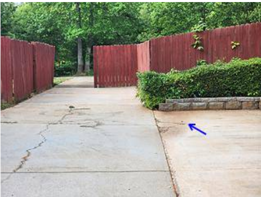
Photo 4-6 Recommend monitoring this area after rain to ensure water is not standing. If standing water is observed have a qualified contractor evaluate and make recommendations for repairs
