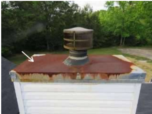
Photo 5-3 The metal chimney cap is corroded, recommend a qualified person prep and paint the cap with anti-rust paint to prevent further deterioration and leaks
