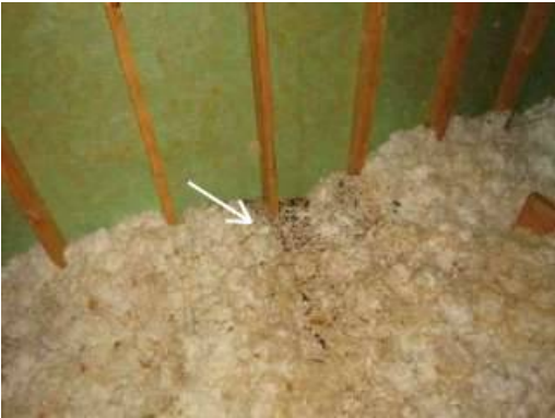
Photo 26-6 Droppings observed below damaged gable screen
