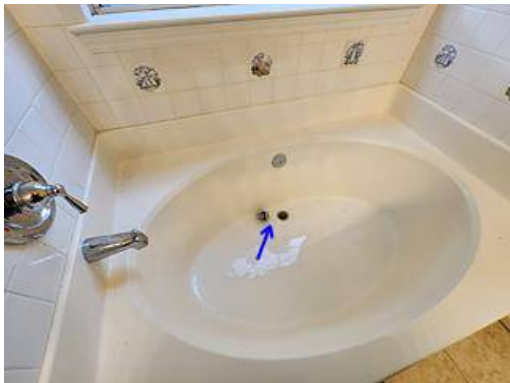
Photo 23-5 Master bathroom drain stopper is detached
