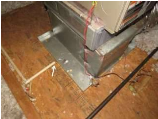
Photo 16-1 Drain pan drain line disconnected from drain pan
