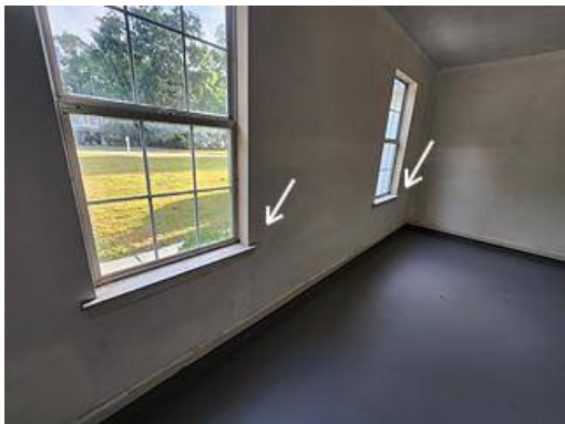
Photo 6-3 Dry stains noted at some window sills, recommend monitoring
