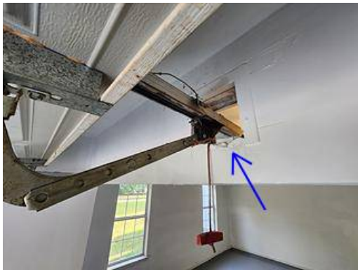
Photo 6-1 The garage door arm hits this area when opening. Recommend a qualified specialist adjusting the opener limit to stop prior to hitting this.
