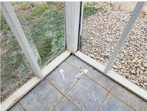
Photo 4-4 Screen loose in some areas
