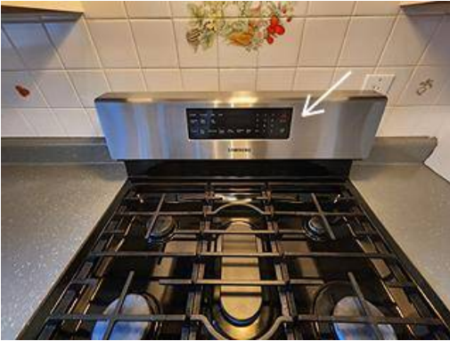
Photo 7-3 The stove was off at the time of the inspection
