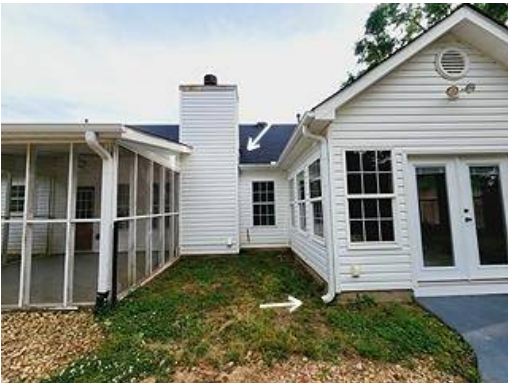
Photo 5-4 Kick-out flashing missing at the chimney area Splash blocks missing
