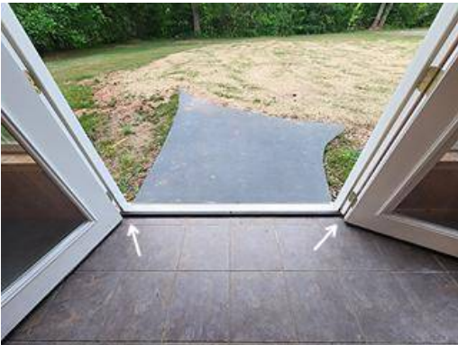
Photo 24-6 Repairs noted, dry stains observed. Recommend monitoring
