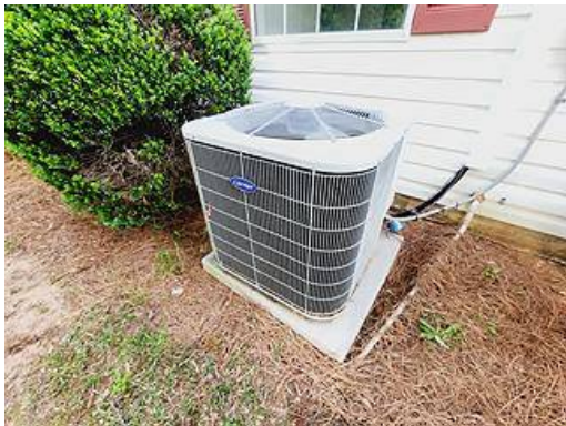
Photo 18-1 Carrier AC unit Left side of home
