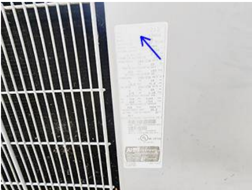
Photo 18-2 Manufactured 2014 3-ton unit
