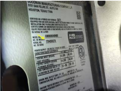
Photo 29-6 Manufactured 2017 Filter at base
