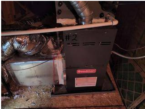
Photo 29-7 Goodman gas furnace #2 Attic location
