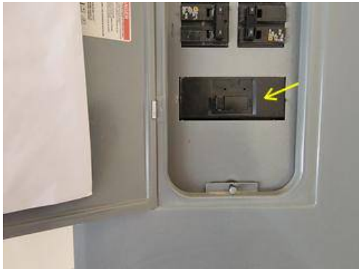
Photo 23-1 Bottom of service panel
