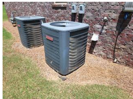
Photo 29-1 Goodman AC unit #1 Left side of home
