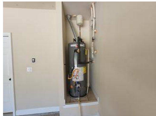
Photo 25-1 Rheem gas water heater Garage location
