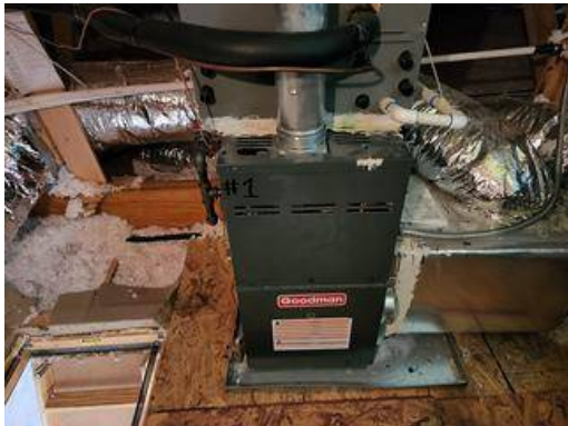
Photo 29-5 Goodman gas furnace #1 Attic location
