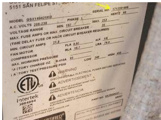
Photo 29-2 Manufactured 2017 3.5-ton unit
