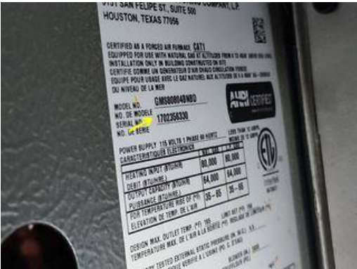
Photo 29-8 Manufactured 2017 Filter at base
