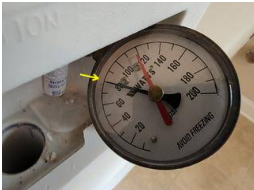
Photo 44-3 Water pressure @ 80psi
